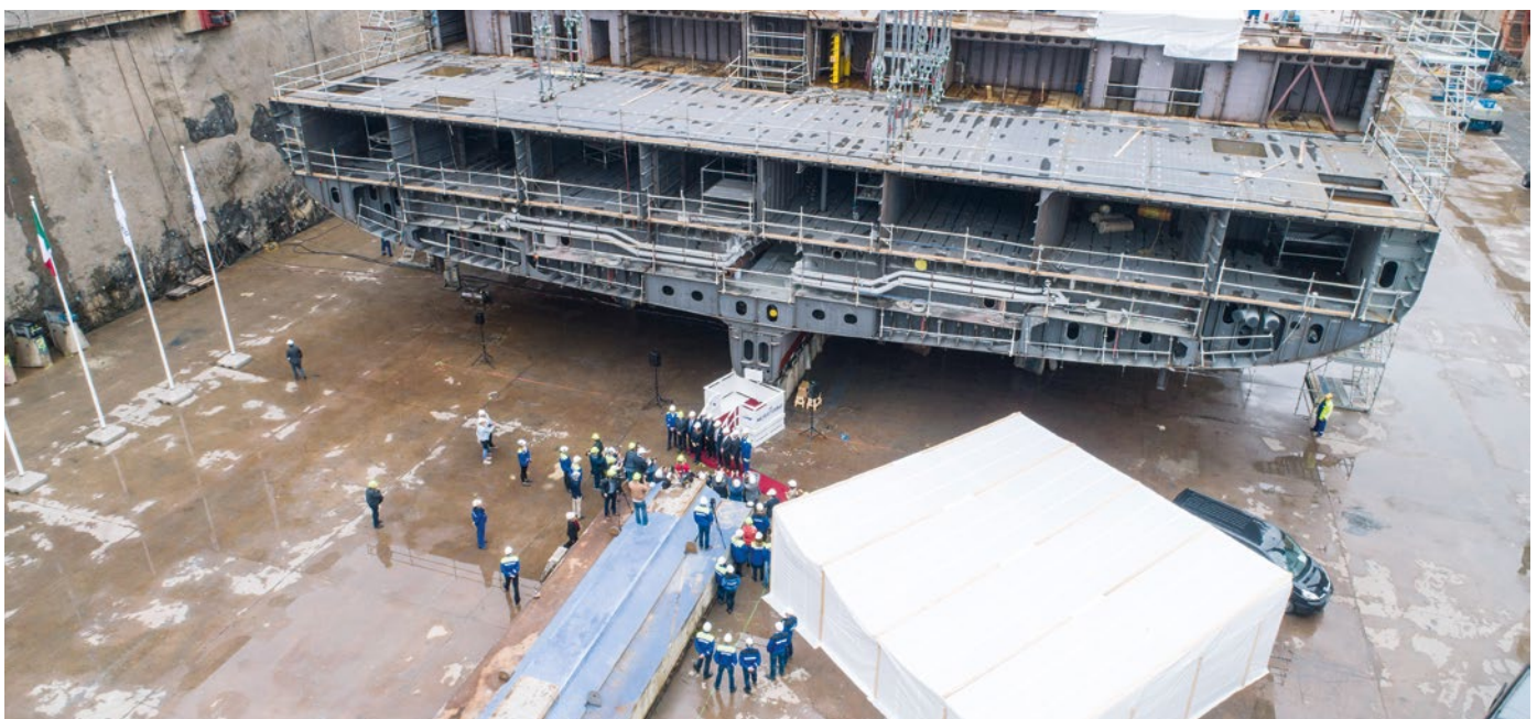
In contrast to the roofed dock in Papenburg, the cruise ships are constructed in full length – from tank to observation deck – in the open docks in Turku.
